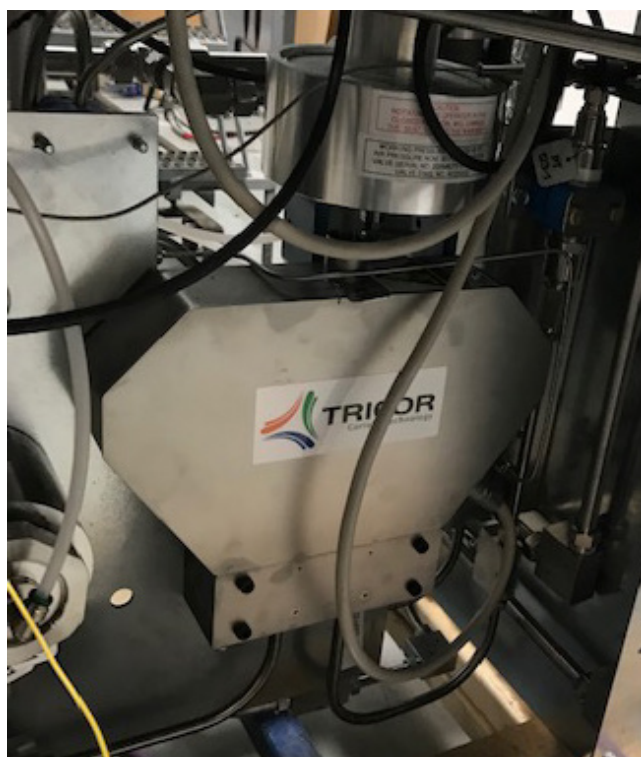
Rear view of hydrogen pumping station showing TCM-0450 High Pressure MID-002 / OIML certified Coriolis meter.
