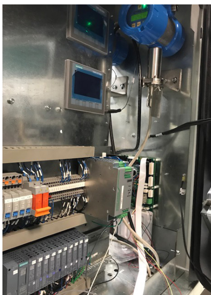
Rear view of control system with IO cards and dispensing controls
